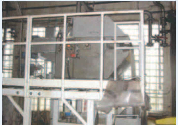
Installation in pulp and paper plant
